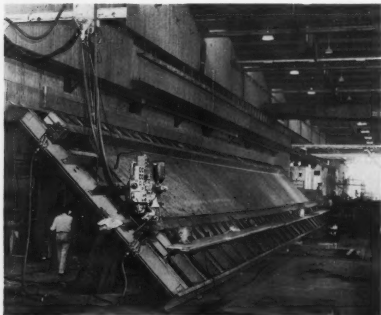
EASY HANDLING: Assembly fixture tilts to welding position. Tractor-type carriage holds tandem-arc unit in the web of the girder.
